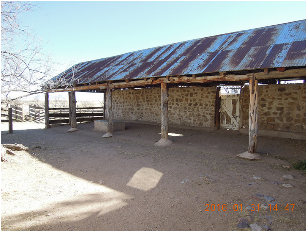
Figure 25. 1870 Stone Corral, Roof Structure Supported by Rough-Hewn Logs. View Looking East. Gina Chorover, 2016.
