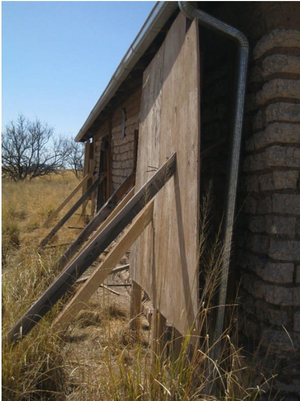
Figure 34. Plywood and Posts Used to Support Unstable Adobe Brick Wall. Taira Newman, 2016.
