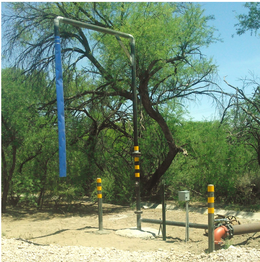
Figure 10. New all-weather water station installed at the Bingham Cienega Natural Preserve in 2017.
