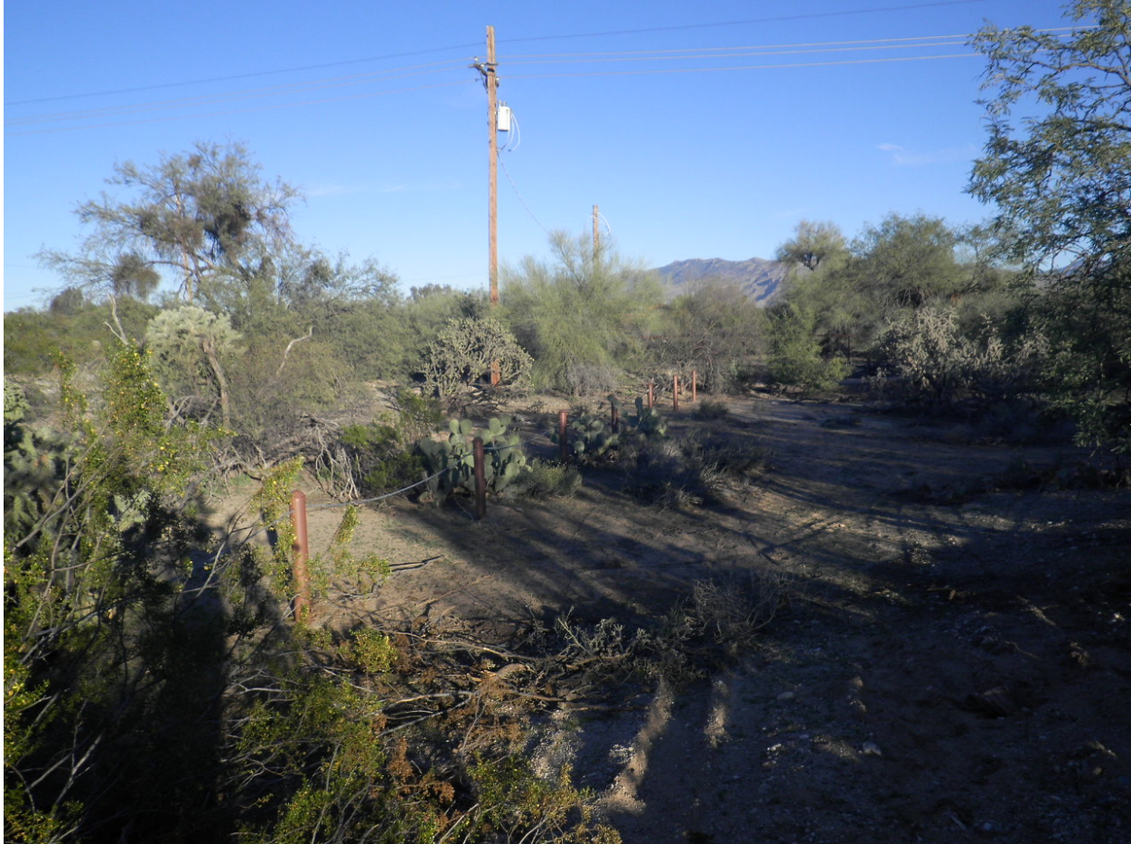
Figure 14. Installation of cable and post to prevent OHV access at an open space property along the Pantano Wash (photo date 12/20/2018).
