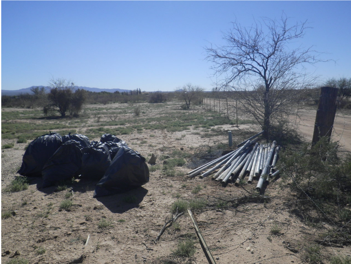
Figure 18. Removing open-topped pipes (a wildlife-trapping hazard) and trash from a County property in the Brawley Wash area (February, 8, 2019 photo).
