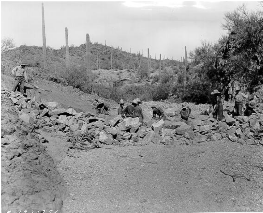
Figure 50. CCC Construction crew at work on Water Conservation Dam, October 1934, Sina Bar Dam, Tucson Mountain Park, Arizona.
